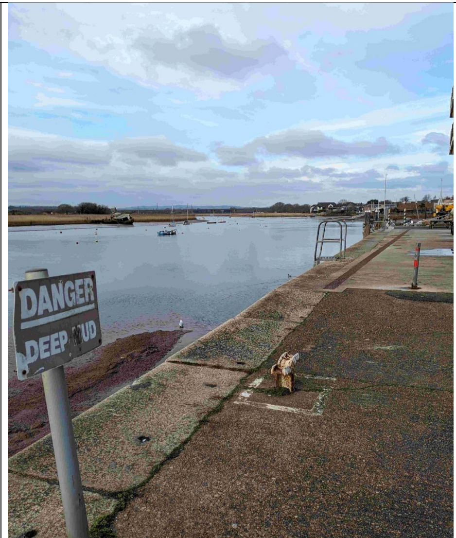
Image B4. Topsham Quay Signage to Review and Bollard Trip Hazard
